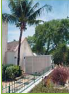
Concealed MBR Plant at a Caribbean Hotel
