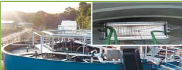
Submerged MBR Module at the Retrofitted WWTP at Bon Accord, Tobago
